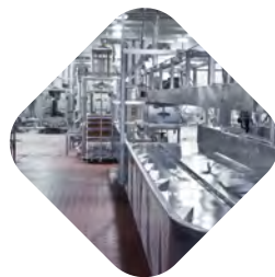
COMMERCIAL DAIRIES & DAIRY PROCESSING PLANTS
